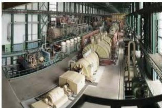
Turbine hall before any dismantling (05/2013)
