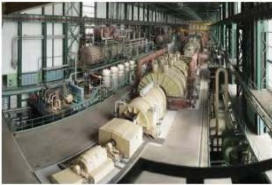
Turbine hall before any dismantling (05/2013)
